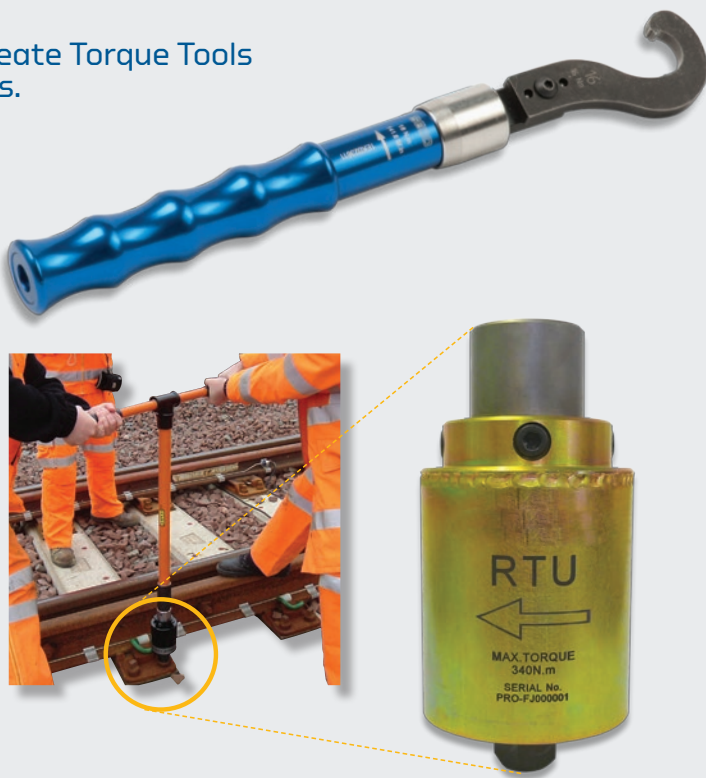
Modification of RTU for Track Bolt Tightening
